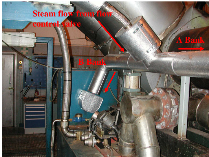
Figure 3.13: a part of the steam injection system at WPPP
